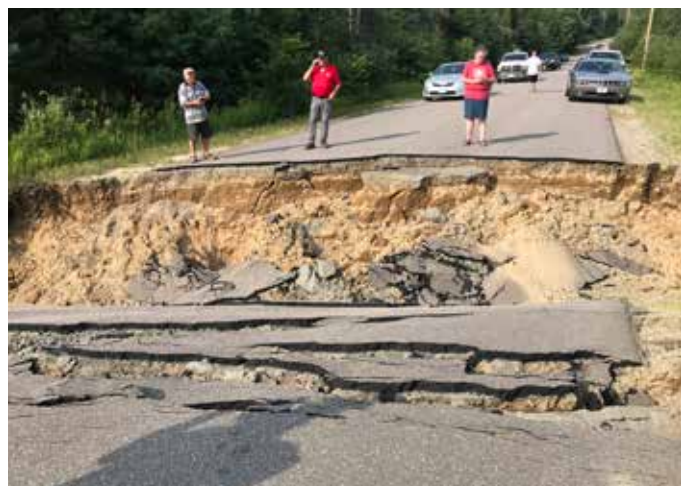
Washout on North Baptiste Lake Road, July 27 causes major repairs. Photo by Paul Coleman
